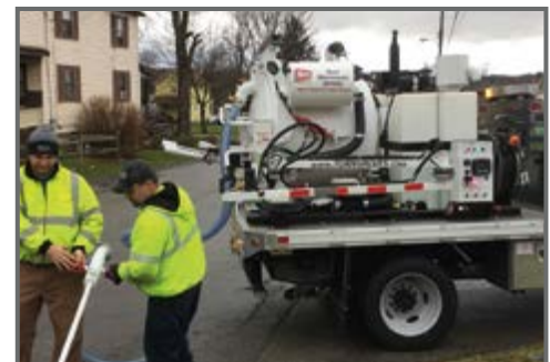
500 CFM Vacuum Pump for valve box clean out
